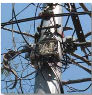
Phone wires connected at the utility pole outside. Where is the cover?
