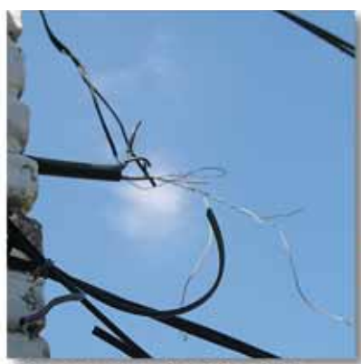
Phone wires leading into the house.
